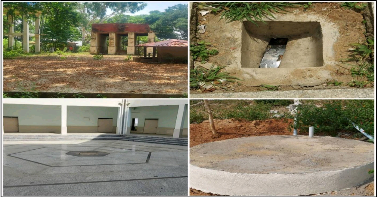
Figure 8. Rainwater harvesting unit, Ground water recharging facilities, Percolation Pond, Water Reservoirs, etc. for storage of water to maintain the ground water level.
